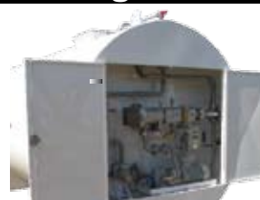
Self-bunded aviation fuel tanks
