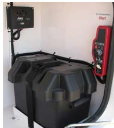
Battery case, electric keystart for compressor and regulator from solar panel
