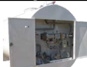
Self-bunded aviation fuel tanks
